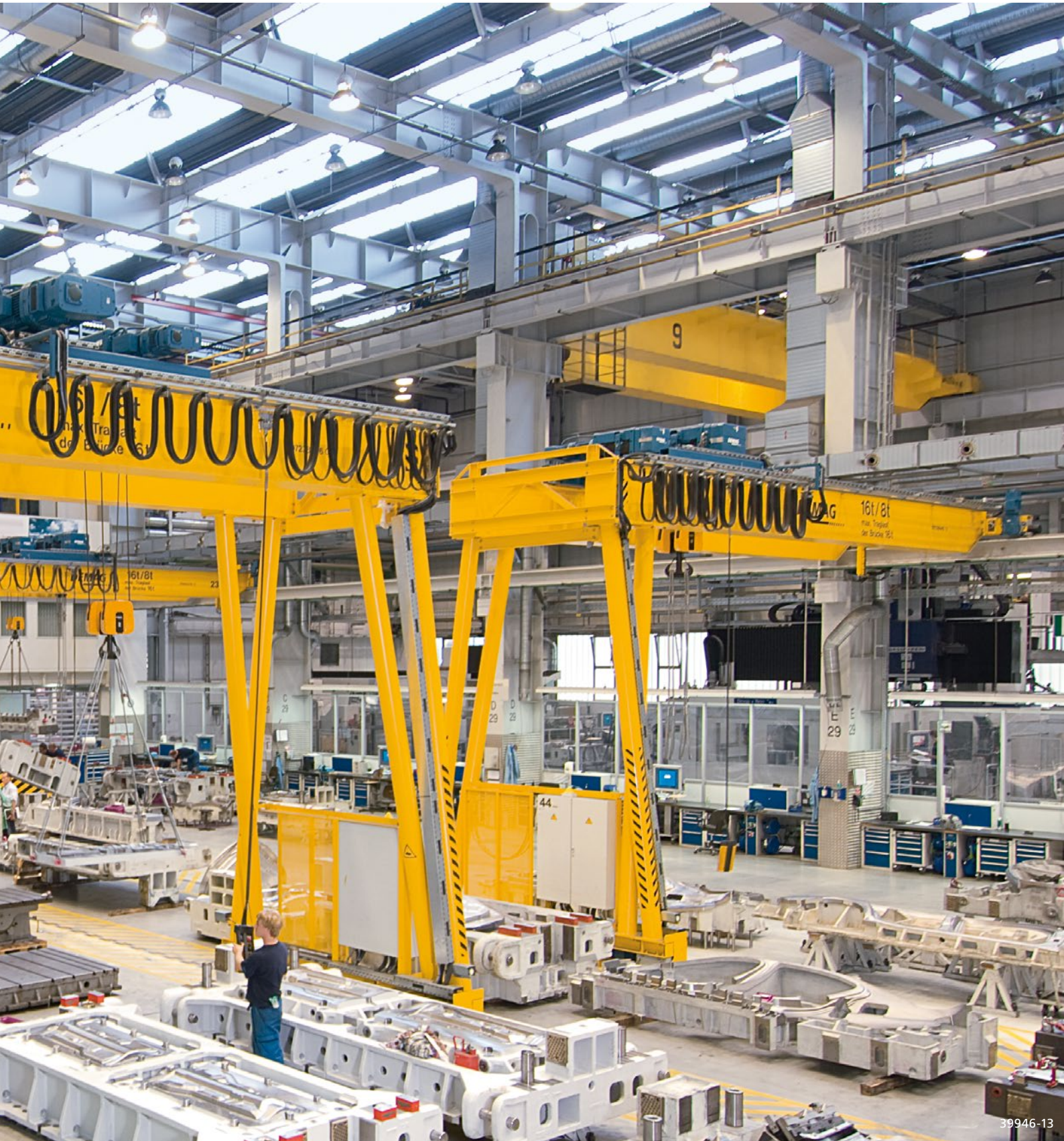
Double-girder semi-portal cranes for maintenance work on press tooling at an automotive production facility
